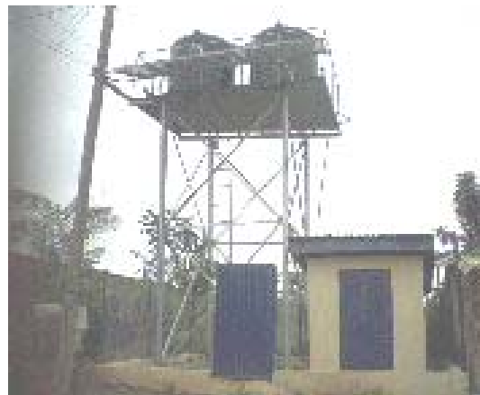
Plate-4. Reticulated solar-powered borehole.
